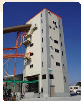
Concrete plant (BP-Related Business)
