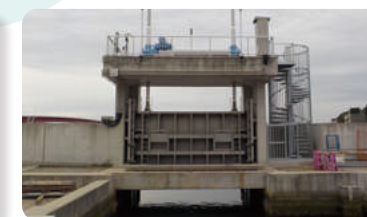
Floodgate (Other Business)
