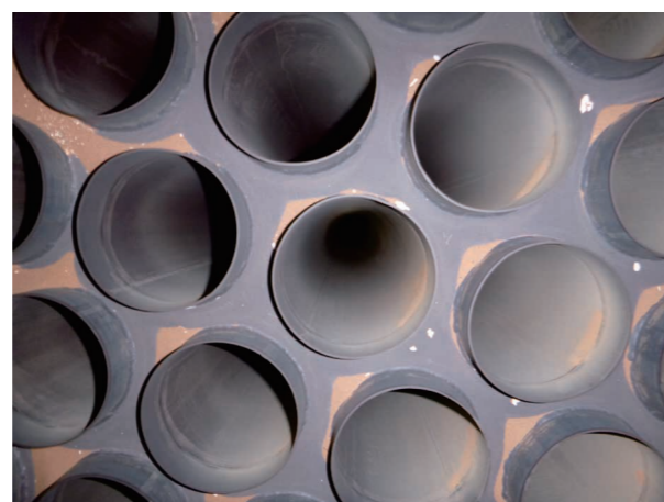
Fig8 inside of the heat exchanger
