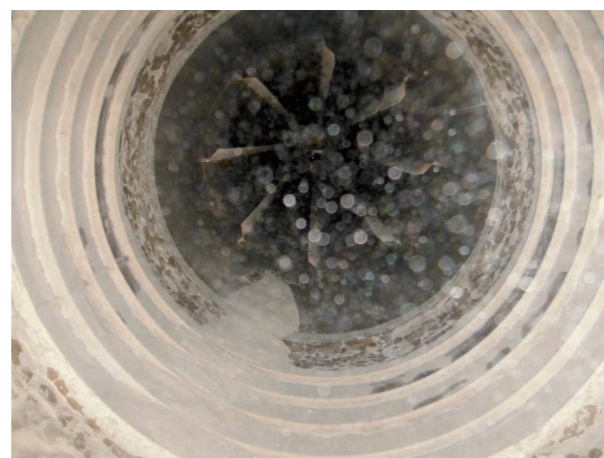
Fig5 inside of the pre-drying device
