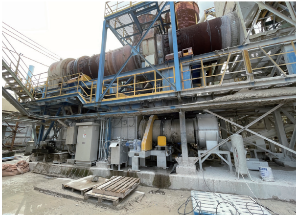
Photo 2-1: Facility for Producing Type-II Anhydrous Gypsum
